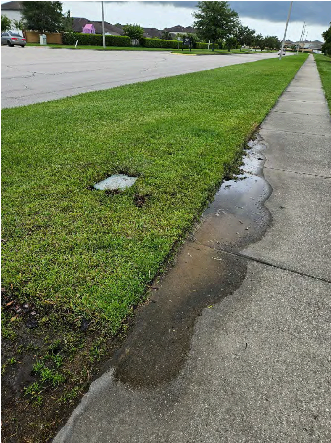
Small mainline leak at valves 36 and 37 on A2C controller.
